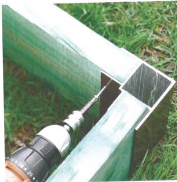
3 Attach boards to metal corner brackets with stainless steel screws. We used six corner brackets and four inline connectors, available in a kit from Gardener's Supply Company.
